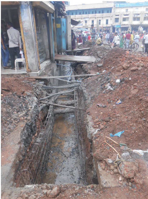
Fig. 3. An open sewage drain opposite the north-eastern wall of the Jagannath Mandir (Photo by author).
